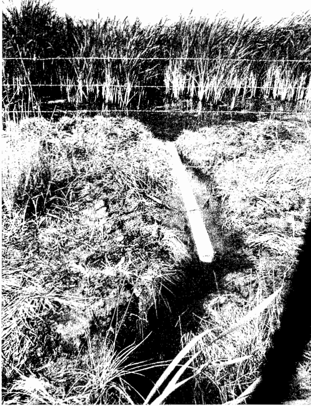
Lateral Pipe draining
